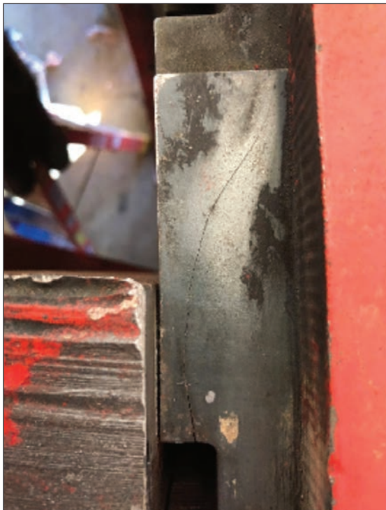
(c) Looking down on a cracked rotor rim lamination next to the shrink key slot.
