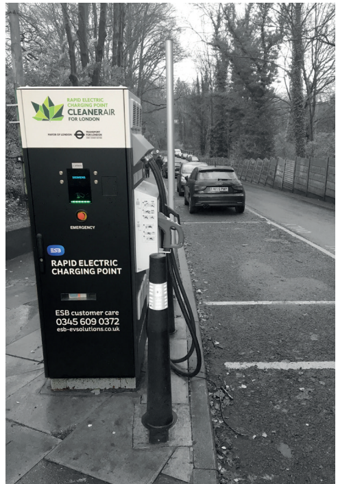
Example of a current EV charging point
